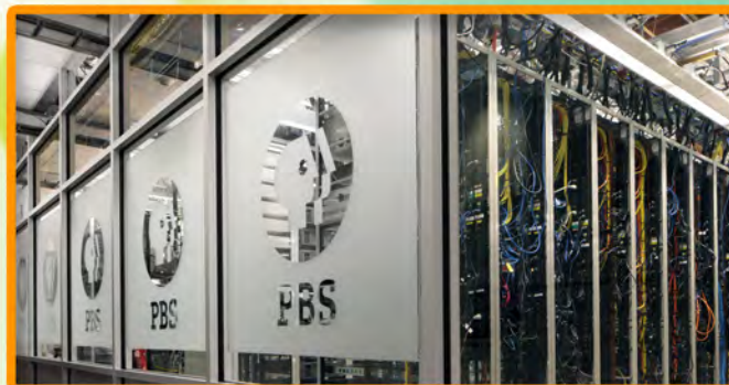
Exterior view of the Technology Center Main Equipment Room (MER)
